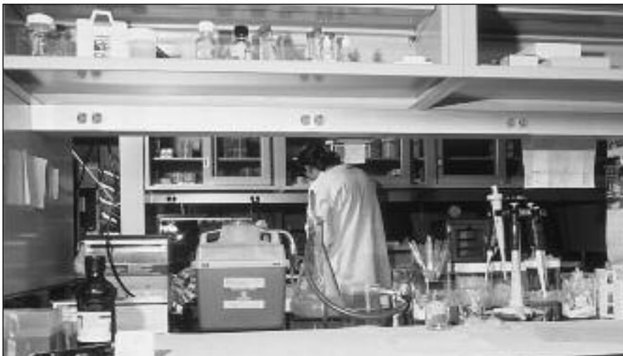
Standard devices installed in aluminum raceway mounted under reagent shelf in medical center lab.
