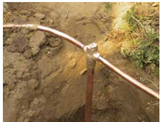
GT Cadweld connection
