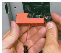
2. Attach the lockout device to the breaker and snap into locked position.
